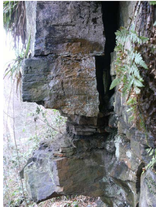
Photo GGS_5 P4: Close-up illustrating how some of the sandstone blocks at this site are hanging very precariously, daylight can be seen through this vertical joint (GGS_5b).
