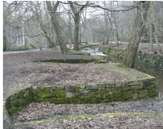
Photo GGS_4 P4: The mill lade which channelled water from the River Kelvin to power the flint mill. The lade bed was cleaned, lined with stone and the walls cut down for safety in the 1970's. The site now forms part of the Kelvin Walkway and lies within the boundaries of the Glasgow Botanic Gardens. Looking NW.
