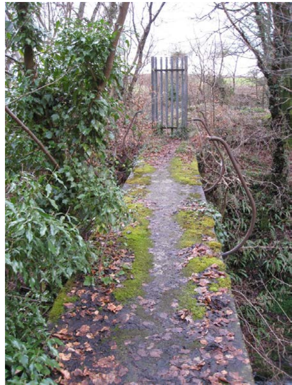
Photo GGS_13 P2: Footbridge across Brock Burn in state of disrepair. This is the only access to sections on the west side of the Glen. Looking W.
