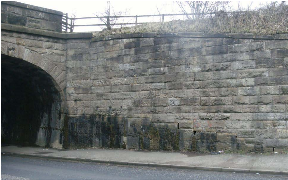
Photo GGS_7 P1: The southern entrance to the tunnel where the Nitshill Road passes beneath the railway line, looking NE. The lower portion of the cutting is in sandstone bedrock, thought to be the Nitshill Sandstone (Limestone Coal Formation). The sandstone unit is described as reaching 20m thick at its maximum, and was extensively quarried in the Nitshill area as a building stone.
