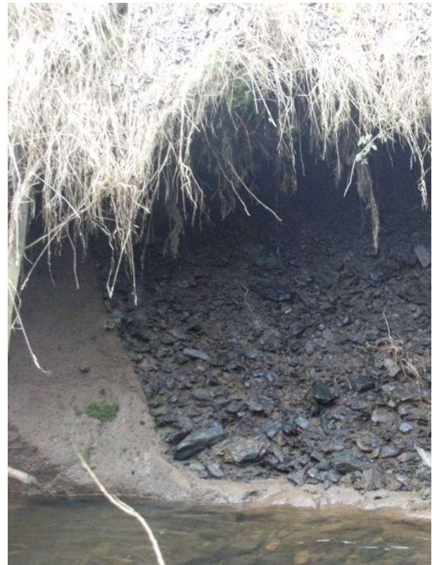
Photo GGS_3 P6: Close-up showing the irregular nature of the base of the made ground and how it cuts down into the underlying natural superficial deposits (GGS_3b). Looking NW.
