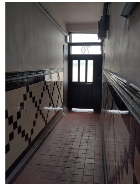
Communal corridor to front external secure access door. There is a large gap between door and unlevelled threshold.
