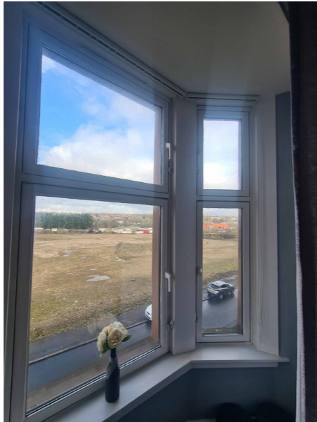
Upper floor flat bay double glazed timber framed windows located on front façade of building.
