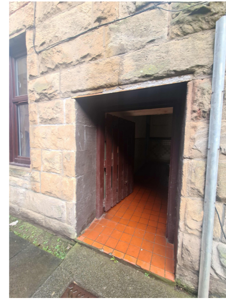
South-facing façade. Erosion found on blonde bullnose ashlar sandstone stonework. Cracked terracotta tile floor coverings on communal corridor.
