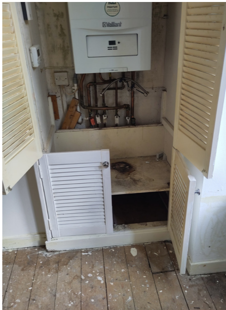
Existing gas-fired combi-boiler providing hot water.
