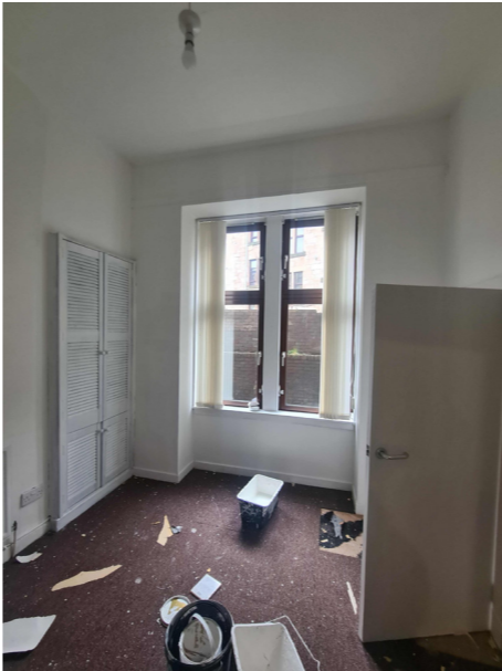
Upper floor flat double glazed timber framed windows located on rear end of building.
