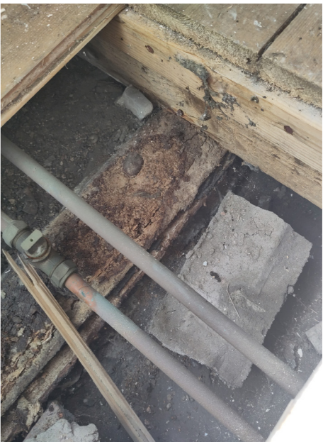
Opening up of suspended timber floor boards to ventilated void revealing timber floor joists and pipework of ground floor flat.
