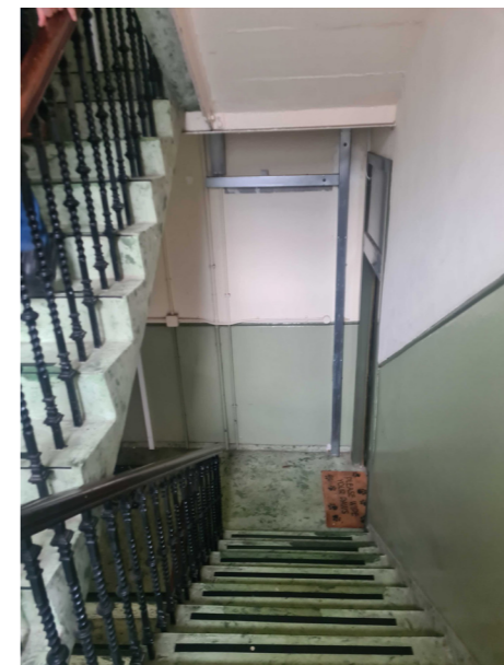
Typical communal stairwell. Cracked terrazzo floor coverings.
