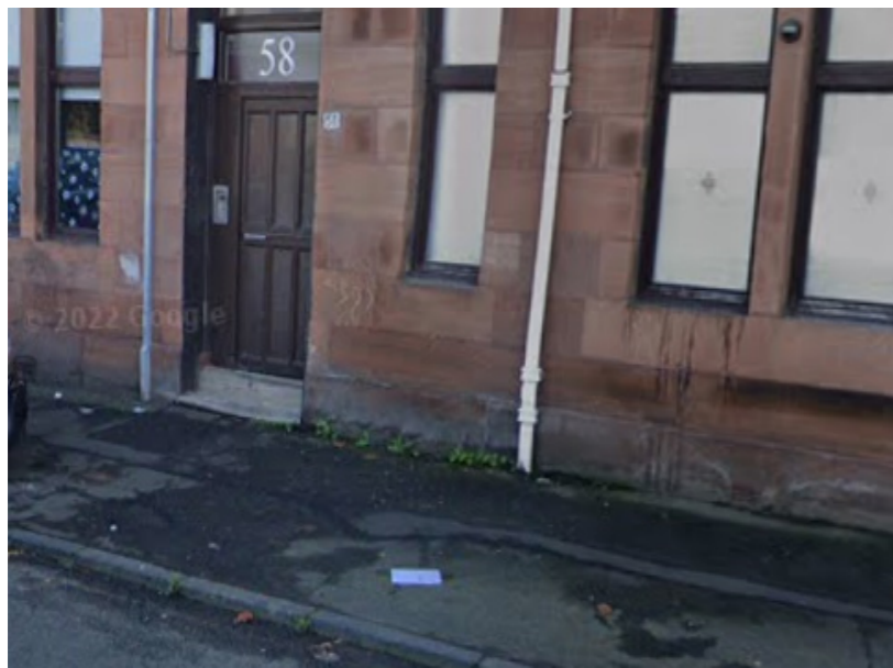
Vegetation growth along base of front façade facing Old Shettleston Road.
