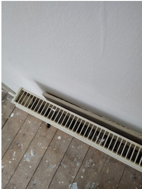
Existing radiators in flat of building.
