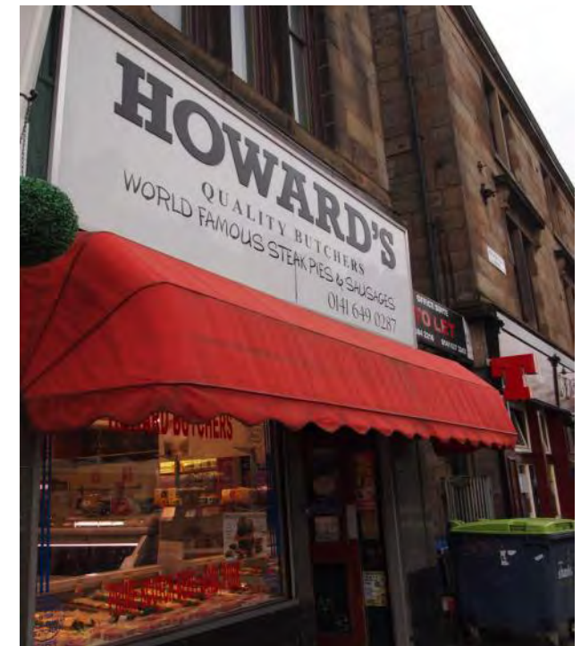
Level 2: Active shops with poor / very poor frontages and window displays, overt security and generally in a poor state of maintenance and repair
