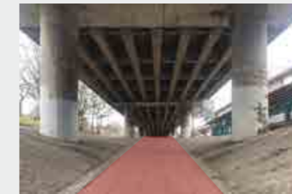
Poor quality and safety of pedestrian passages
