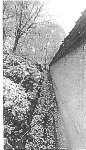
View along south wall of Fossil Grove building showing leaf build up and previously excavated channels
